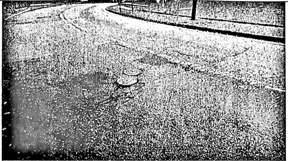
Settlement cracking evident in asphalt surface on Section 1 of Parkvale Drive
