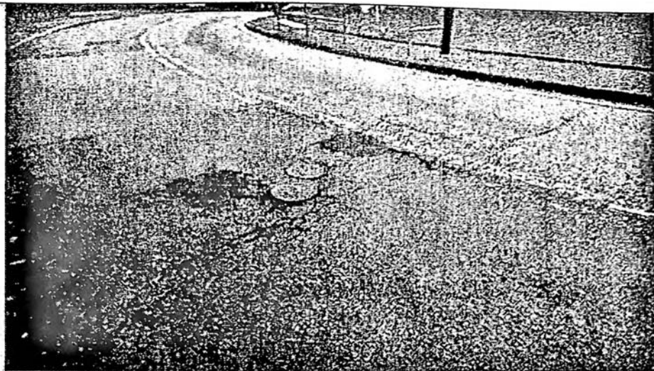
Settlement cracking evident in asphalt surface on Section 1 of Parkvale Drive
